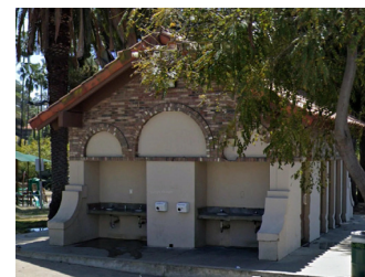
LA SAN managed restroom (2/2)
