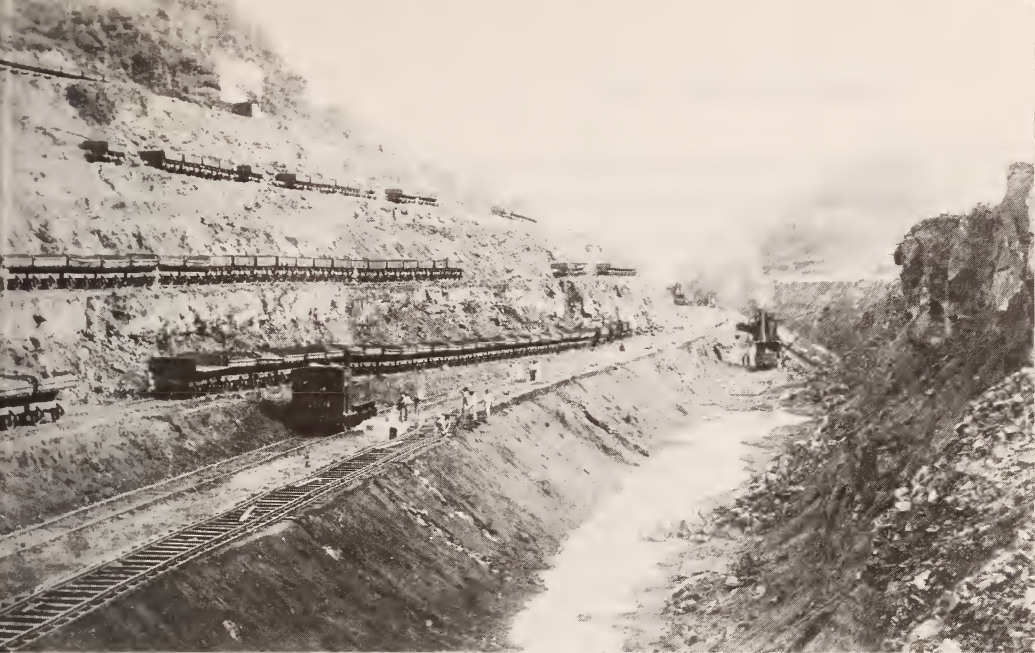
Excavation for the Panama Canal at the Culebra Cut, December 1904 Courtesy National Archives
