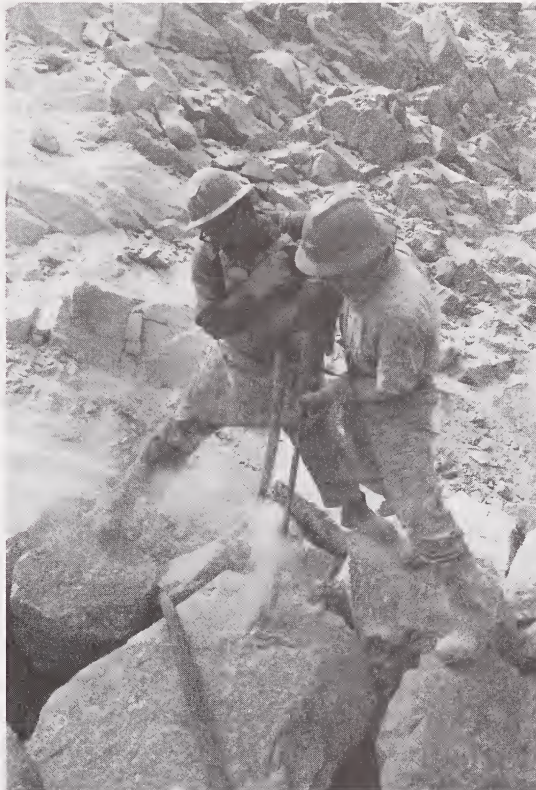
Miners drill dynamite holes at the Mina Raíl open-pit copper mine near Arequipa. Courtesy Inter-American Development Bank
