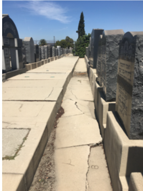
Figure 5.1: Cracked Concrete in Agudath Achim. Photo by author.
