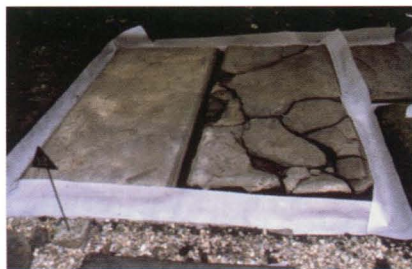
Fig. 2. Emergency stabilization by means of temporary reburial with sand and geofabric "pillows." Photograph by Frank Matero.
