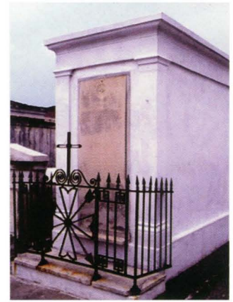
Fig. 10. Perrault Tomb, after. Partial restoration through repair of roof and missing stucco. Photograph by F. Matero.
