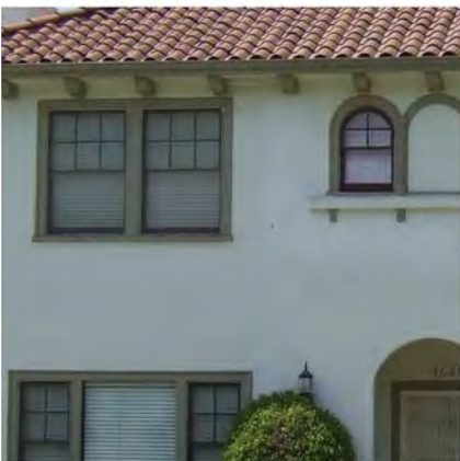
Flush, frameless, and oddly arranged windows may be inappropriate on a new house.
