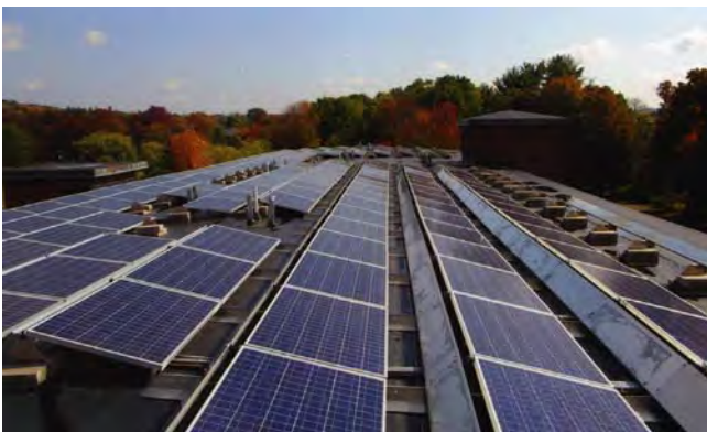
Solar panels installed on the flat roof.
