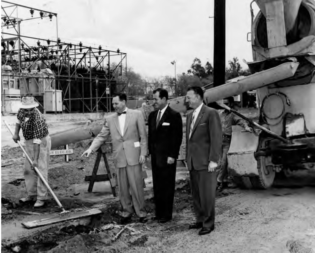
Figure 2.10: Widening a stretch of Van Nuys Boulevard in newly-rezoned business area of Pacoima is inspected by Ben L. O'Brien, Pacoima Chamber of Commerce president, left; William E. McCann, Los Angeles Board of Public Works; and, D.P. Loomis, banker. Source: Valley Times Collection, Los Angeles Public Library.
